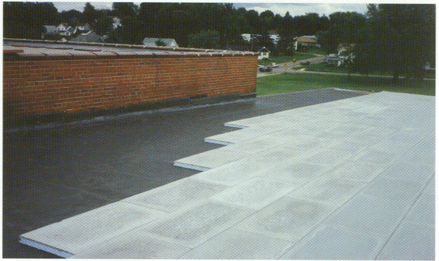
Markesan Middle School in Markesan, Wisconsin. This system, using a single-ply membrane, was applied directly over an existing BUR. At 4.5 lbs./sq. ft., Lightguard can save tear-off costs in most applications.
