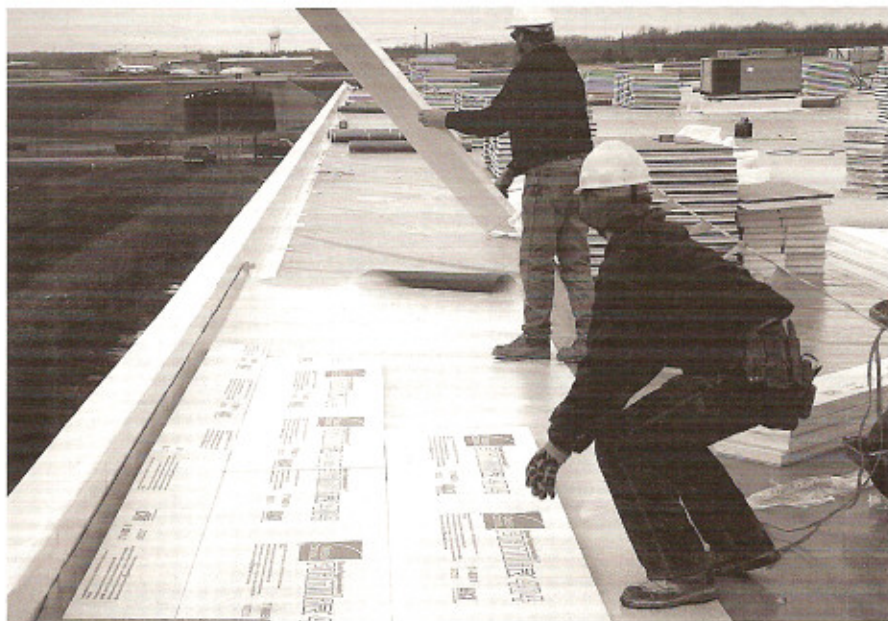
Workers from Progressive Roofing, Inc. are exposed to the wind and cold as they install this Heavyguard Protected Membrane Roof System.
